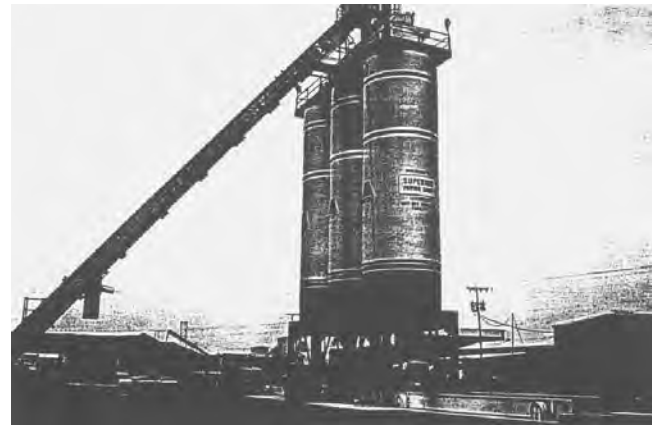
FIGURE 11-1 Slat conveyor feeding silos at an HMA plant.
