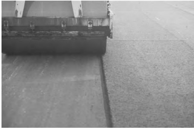
FIGURE 17-14 Starting compaction of longitudinal joint from the cold side, no longer a recommended practice.
