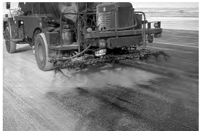
FIGURE 14-8 Improperly adjusted distributor.
