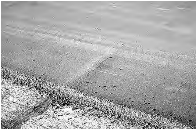
FIGURE 14-4 Bump caused by use of excessive crack sealant.
