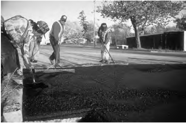
FIGURE 17-7 Excessive raking of transverse joint.
