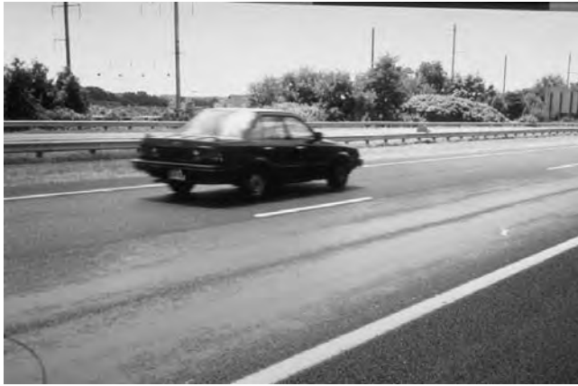
FIGURE 19-8 Fat spot caused by localized excess asphalt.
