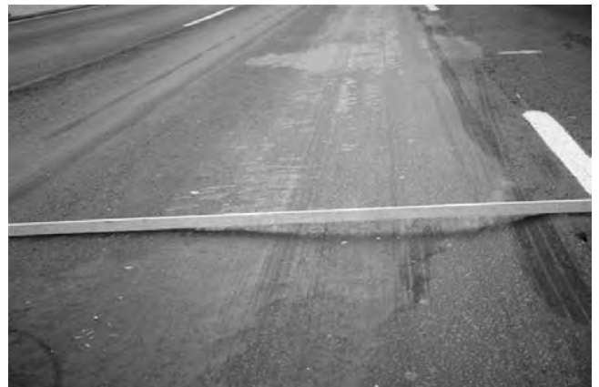
FIGURE 19-6 Rutting of unstable asphalt mixture.
