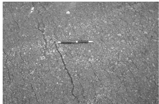
FIGURE 19-4 Hairline cracks caused by roller checking.
