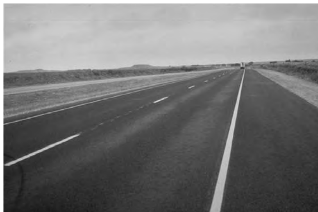
FIGURE 19-7 Asphalt bleeding in travel lane.
